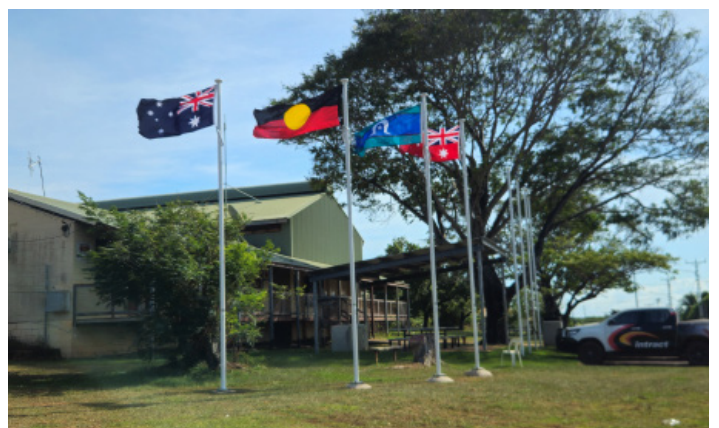
New flag poles have been installed in Minjilang.
