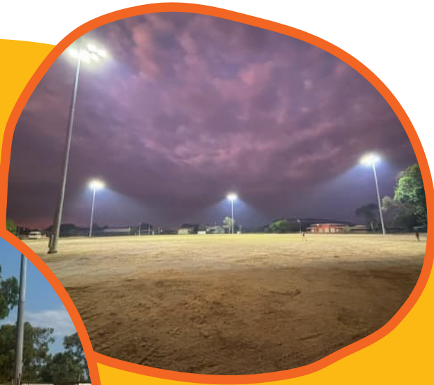
New lights installed on Gunbalanya's Oval.
