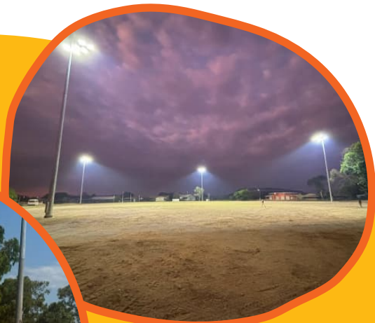
New lights installed on Gunbalanya's Oval.
