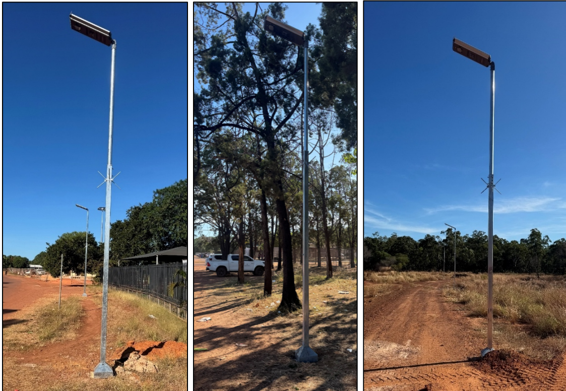
Newly installed Maningrida solar lights.
