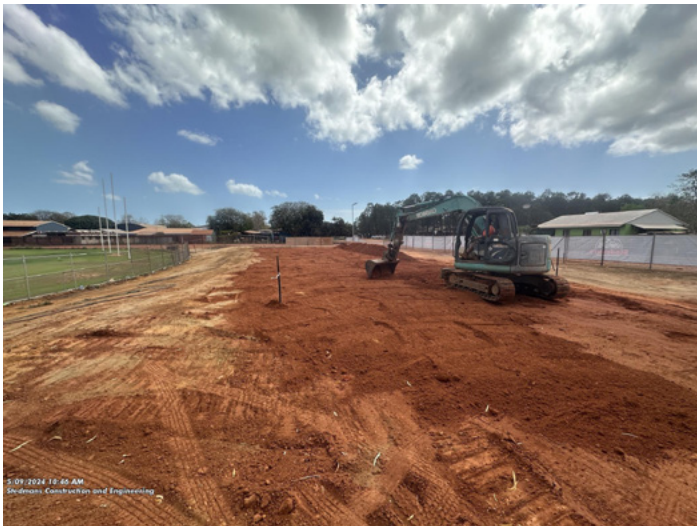
The Maningrida Oval grandstands and changerooms are significant projects which will bring huge benefits to the Community.
