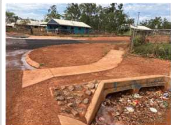
Rubbish and silt in culverts
