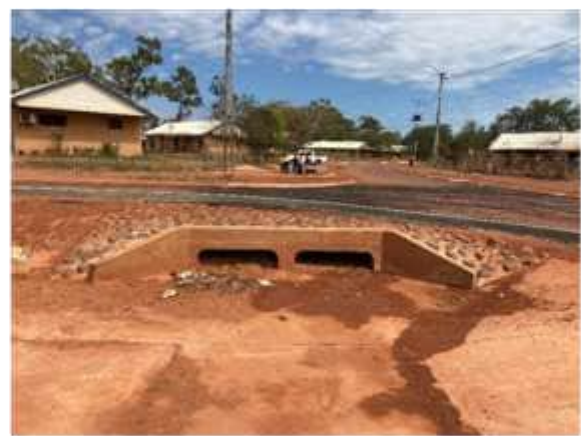
Silt in Culvert TD02
