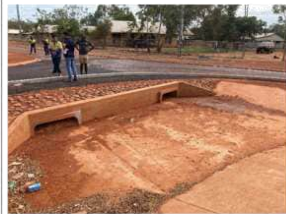
Silt in Culvert in TD02
