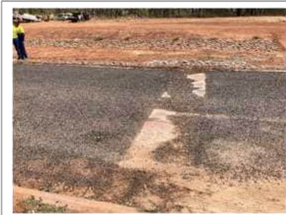
Example of excess stone in invert drain on road A
