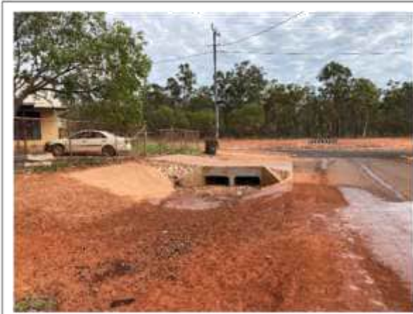
Loose aggregate at the intersection of Road 1 and Gapuwiyak Rd
