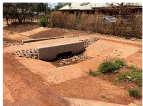
Rubbish and silt in culvert
