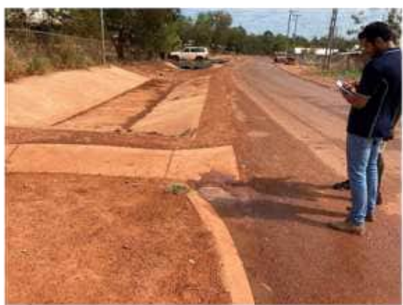
Water ponding between kerb and footpath at intersection of roads C & G
