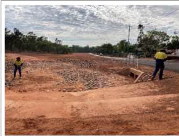
Example of silt in stone pitching at TD02 outlet
