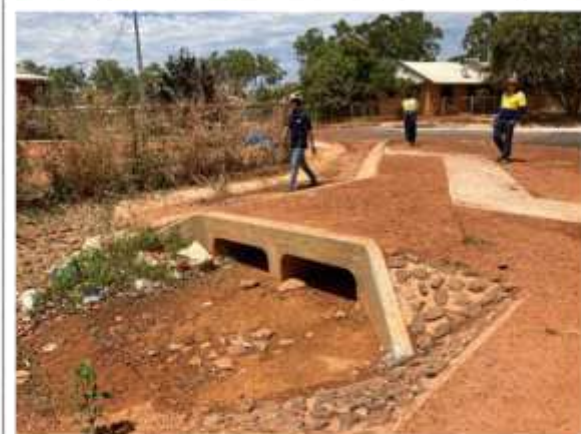
Silt in stone pitching TD04
