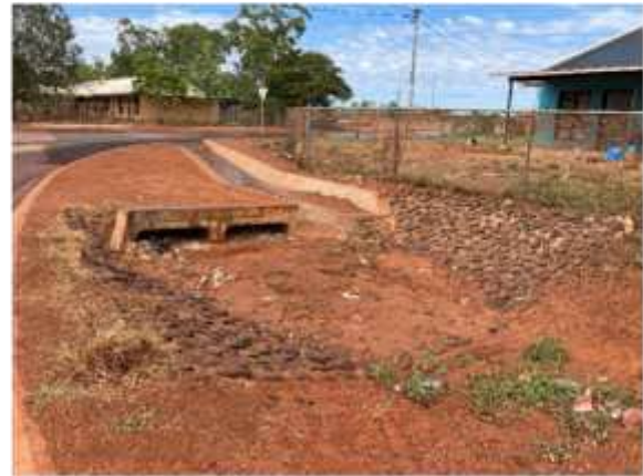
Silt in stone pitching TD02
