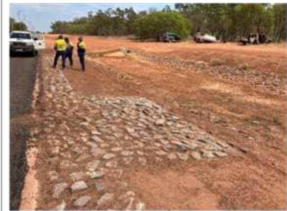
Silt in stone pitching at TD03 outlet
