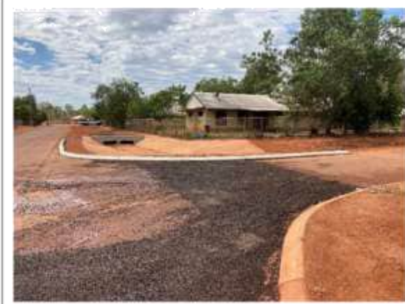
Loose aggregate on intersection of Road C & G
