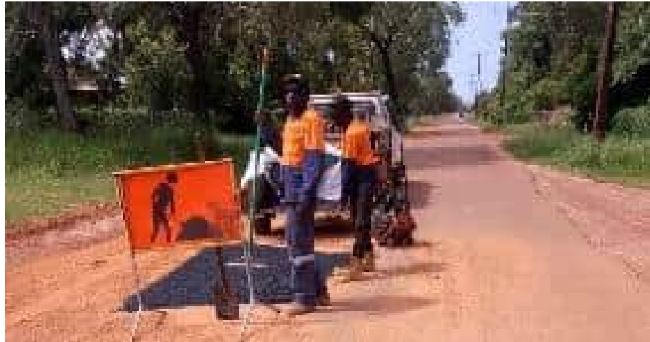
Maningrida Works staff busy mowing the airstrip and filling in pole holes.
