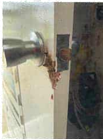
Damaged around door handle
