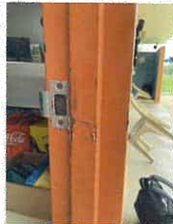
Damaged door frame
